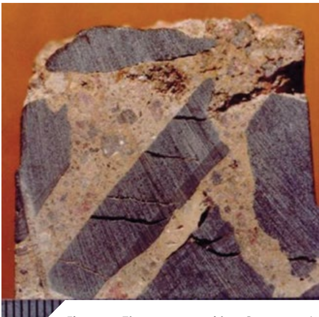
Figure 2: The enemy outside – Damage to the near surface zone of concrete on which sodium sulphate was regularly spilt in a production process (the scale at the bottom of the picture is in mm).
