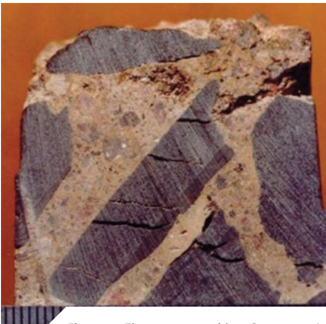
Figure 2: The enemy outside – Damage to the near surface zone of concrete on which sodium sulphate was regularly spilt in a production process (the scale at the bottom of the picture is in mm).
